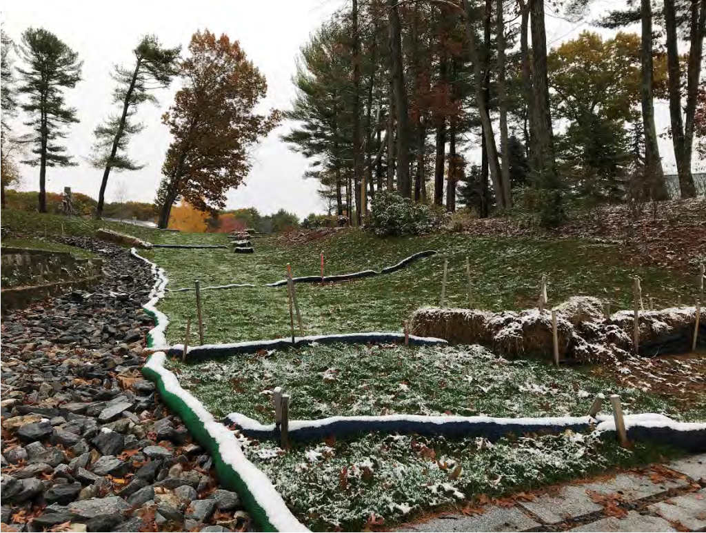
Fig 3: Slope above the manhole at Gundalow Landing/east side of the bay. Viewing east. (10-30-20)
